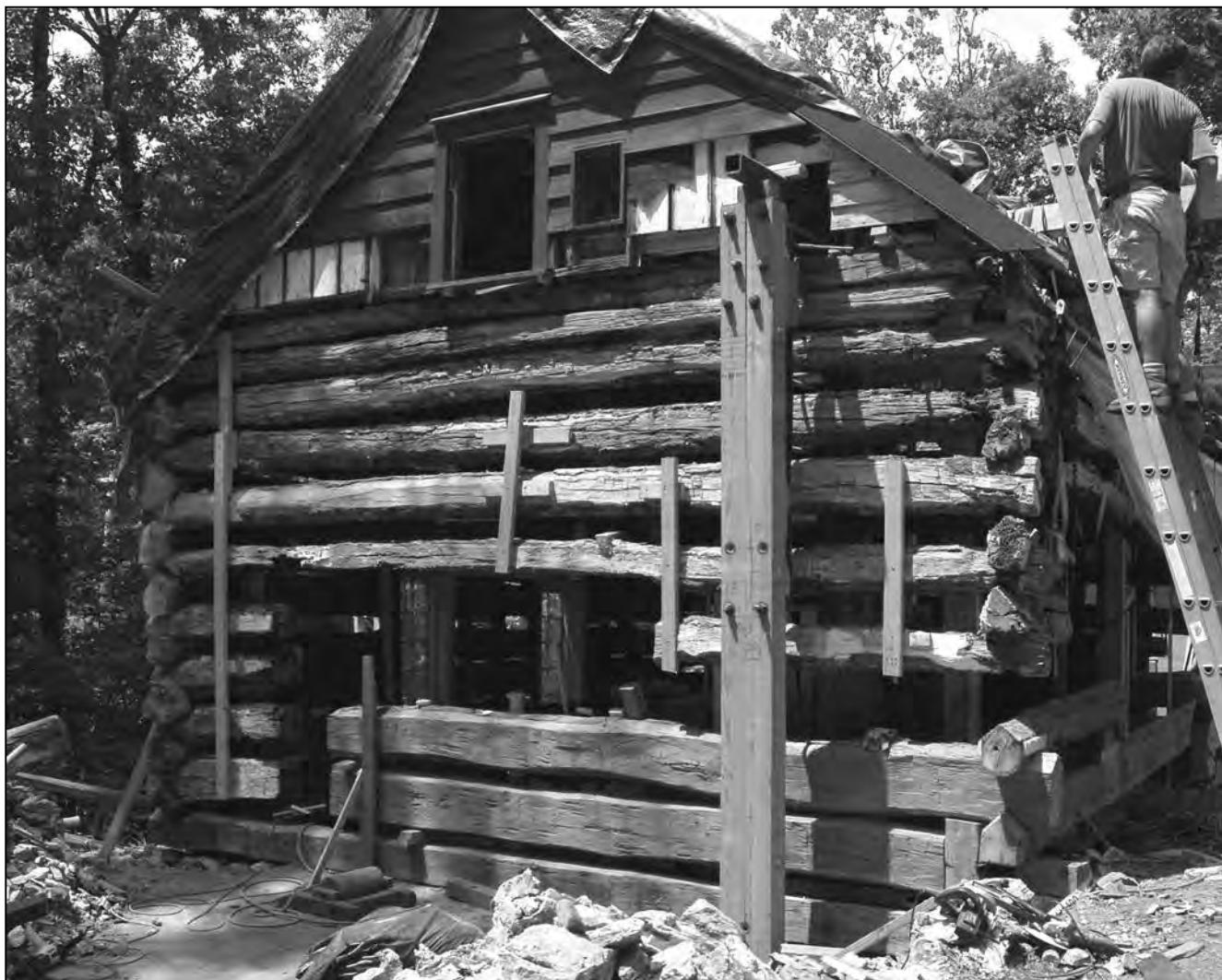
The south wall of the "Church Road Cabin" during its reconstruction. This image, taken July 18, 2008, shows the replacement of the lower logs, all ravaged by insect damage. Many of the upper-level logs were able to be retained despite their age. Courtesy of Roger D. Thorne.
