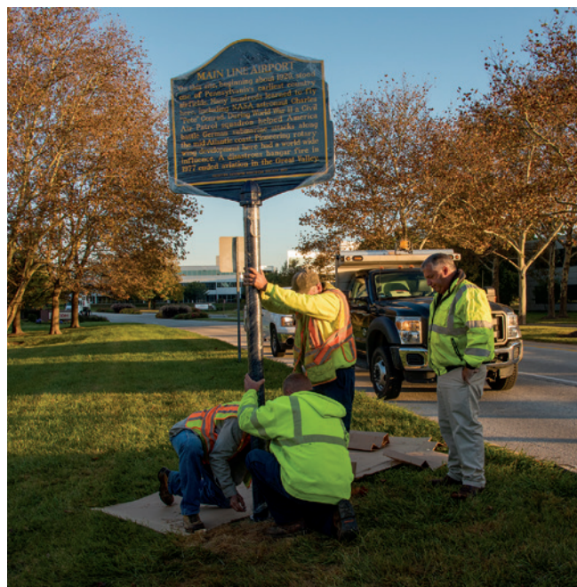
An East Whiteland Township Public Works crew works to install the new marker at the commemoration site on Valley Stream Parkway in preparation for the dedication ceremony to be held two days later, on October 5, 2017. Courtesy of Roger D. Thorne.
